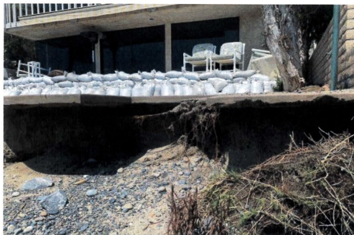
Figure 3. August 2021 photograph of the site prior to the installation of the large sand bags. The actual residence foundation is located just behind the small sand bags and in front of the patio chairs.
