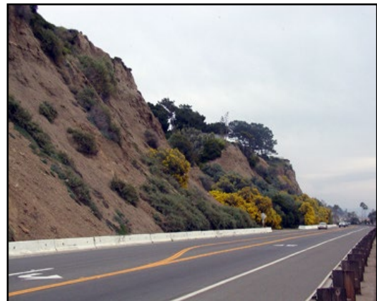
The instability of the Capistrano Bluffs is an ongoing concern. Regulations require development to be adequately set back from bluff edges, and traffic below to be protected from potential landslides.
